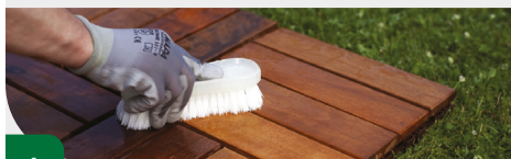
4 After about half an hour, clean with plenty of water removing all traces of the product with the help of a brush with hard bristles.
